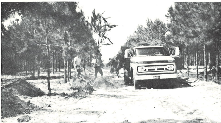
Work nears completion in the Pine Orchard. Campers will be pleasantly surprised when they see the wonderful facilities that have been constructed!
